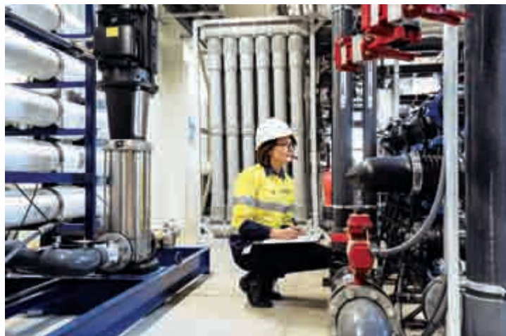
改换用途后改建为“绿色基础设施中心”内的污水处理设施 Water Treatment Facility inside the "Green Infrastructure Centre", a Repurposed Former Hospital Building
