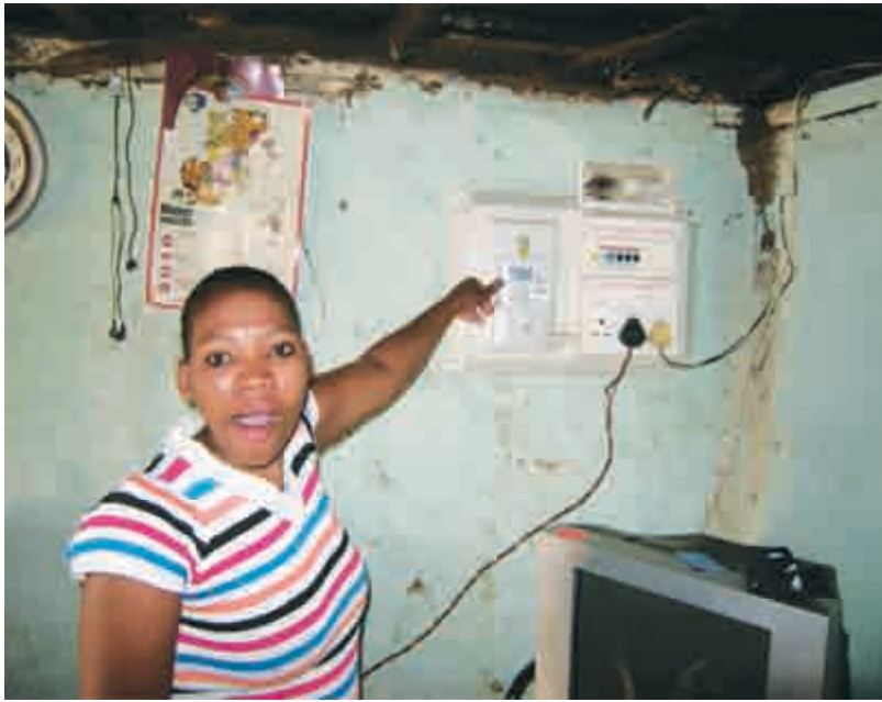
非正式居住区里的个人电路连接 Individual Electricity Connection inside an Informal Settlement
